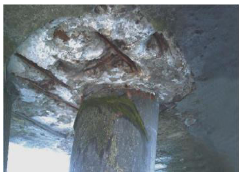
Deterioration of Concrete Structure
